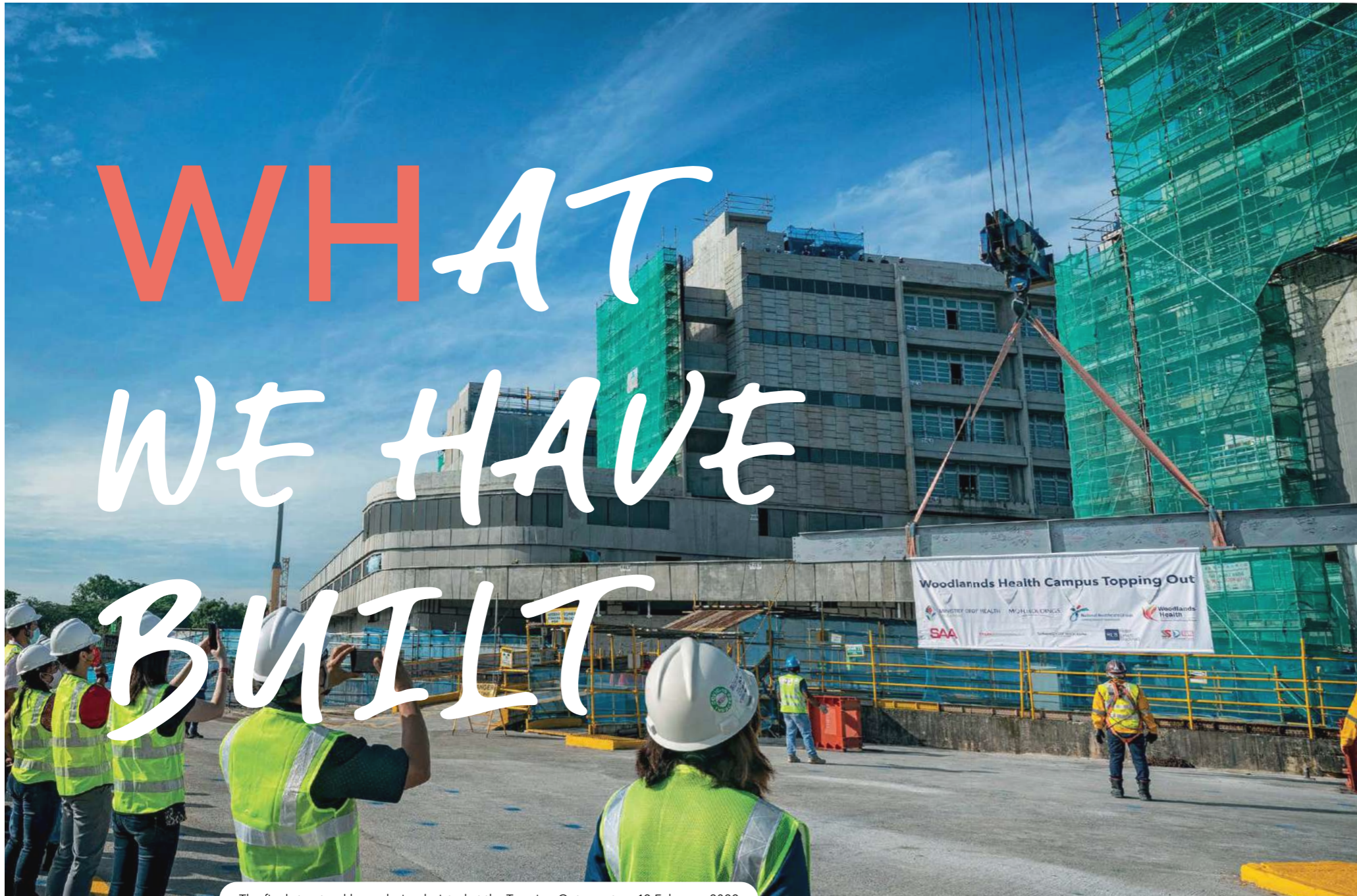
The final structural beam being hoisted at the Topping Out event on 12 February 2022.
