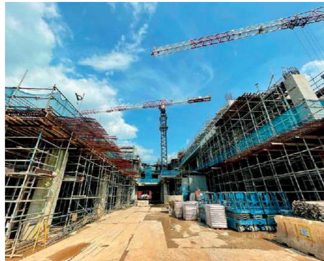
A tense moment for us, when construction came to a halt due to the COVID-19 Circuit Breaker.
